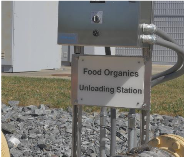
Truck Offload Stations
