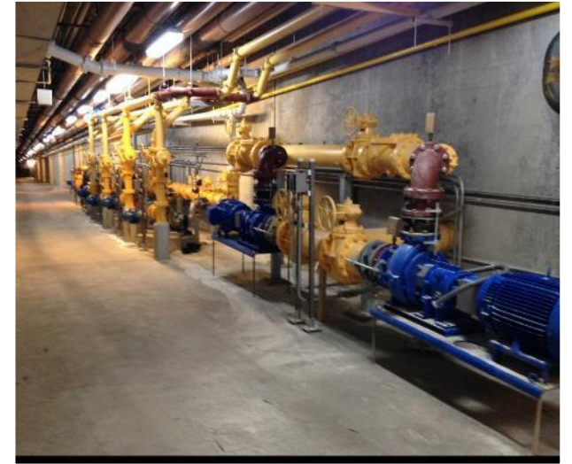
Transfer & Mix Pumping Station
