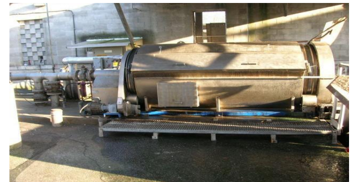
Trucked waste screen at Iona Island WWTP
