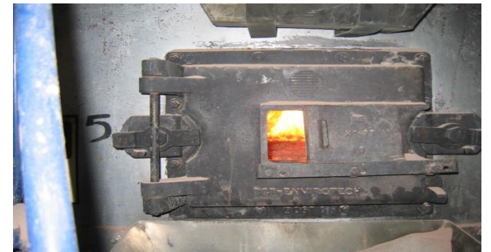
Multiple hearth incinerator at Post Point WWTP
