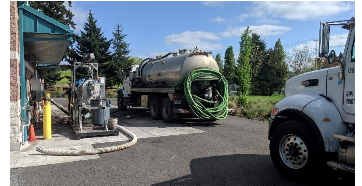
FOG being unloaded at Clean Water Services FOG Station
