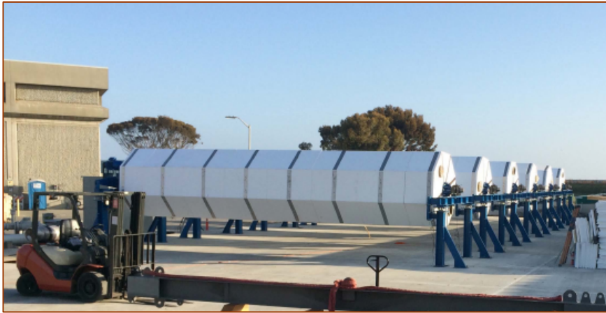
Silicon Valley Clean Water, CA – Biological Drying + Pyrolysis Courtesy: BioForceTech Corporation
