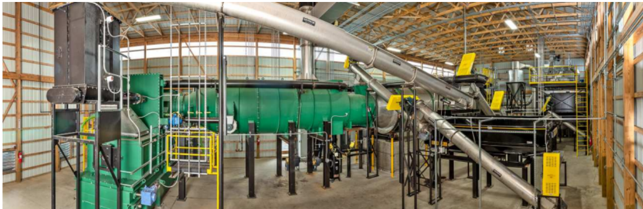
Morrisville, PA – Drying + Gasification Courtesy: Ecoremedy, LLC
